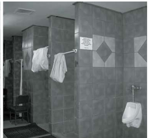
Women could only access showers at specific times and had to cross a public lobby and enter the men's area to do so
