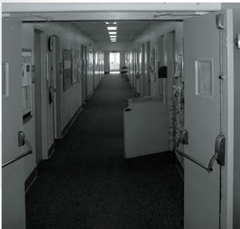
Double doors meant to separate the women's wing from the men's wing were kept open
